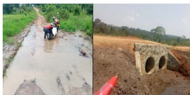
Flooded section of Buwanda swamp in Kalungu district (left) and after works the road was raised, filled with murram and culverts installed allowing all seasonal access
