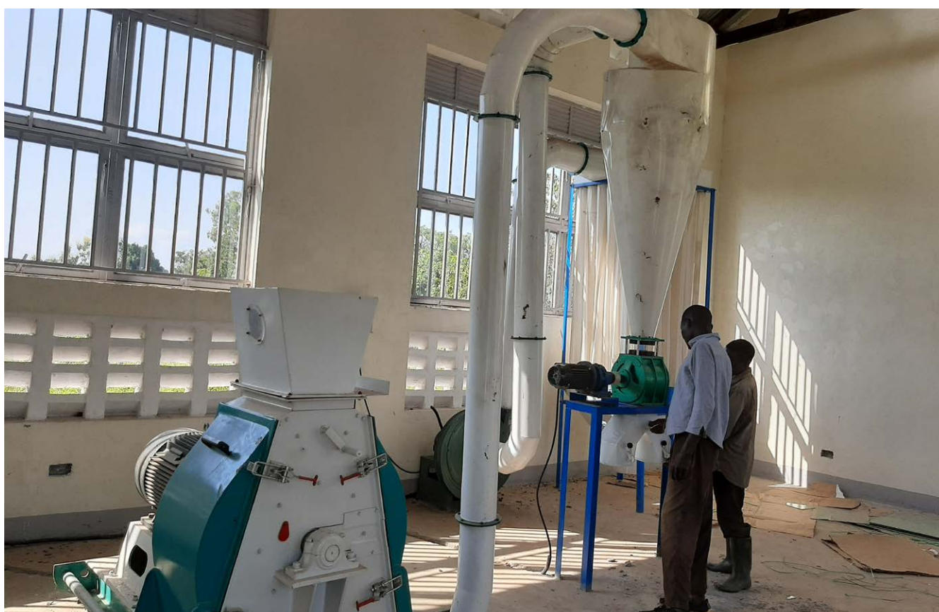
Cassava processing facility (hammer mill capacity of 1-3 tons/hour) installed at Aliamu Cupiria Timbakua Seed development association (ACTS)
