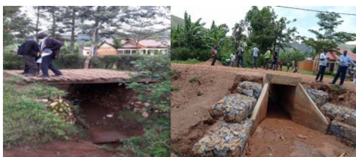
(before) Improvised crossing on Omugenyi – Ahamuyaga Road in Ntungamo (After) Constructed Box culvert
